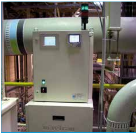
RefillMatic control unit
