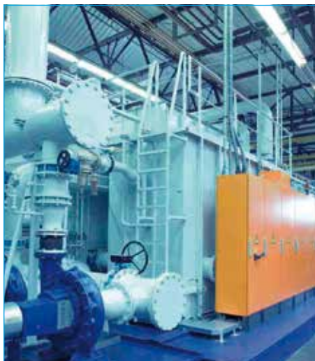
Control cabinet and pump supply
