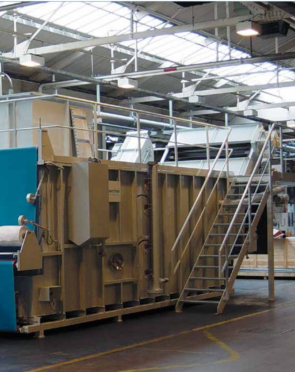
Vacuum filter facility with Viavent pump system
