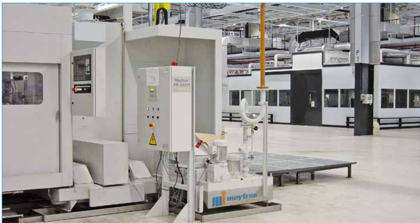
Machine pump station directly on the machine with supply to the Viavent overhead system
